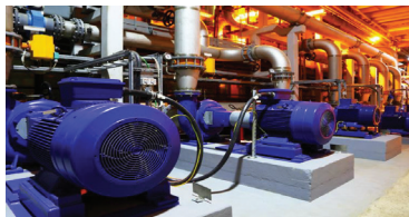
Figure 1. Company with electric motors
