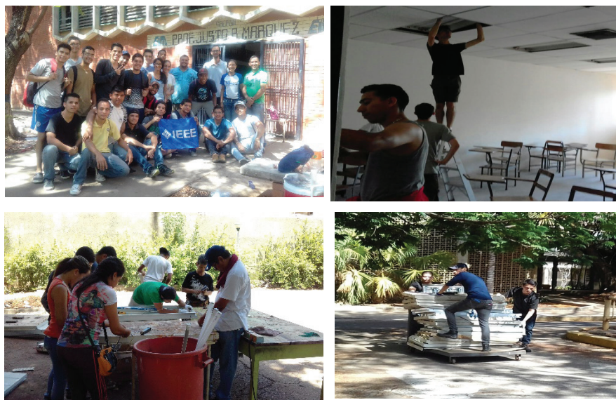
Figura 1. Restoration and replacement of luminaries in the Engineering Faculty of the Universidad del Zulia as part of the “Una mano por tu Facultad” project.
