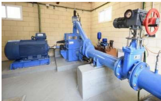
Fig. 3. Pelton-type hydraulic turbine and 60 kW asynchronous electric generator.
