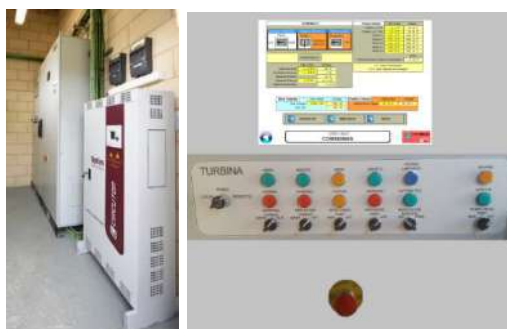
Fig. 4. Capacitor bank and turbine control panel.
