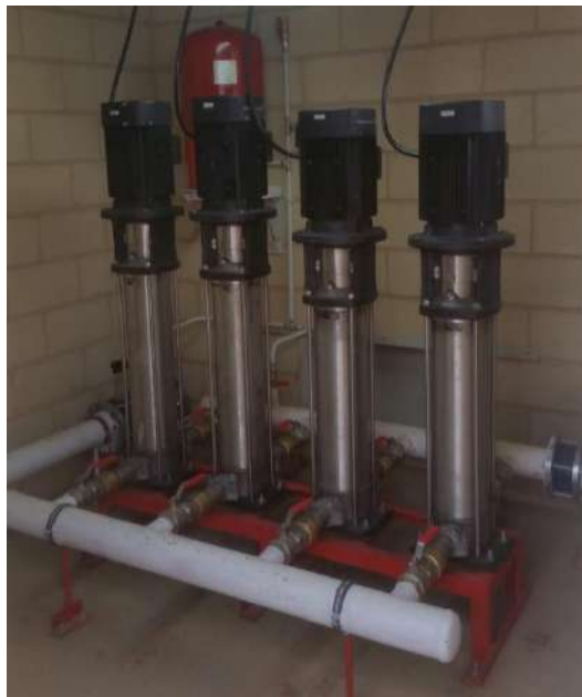
Fig. 14. New pumping system
