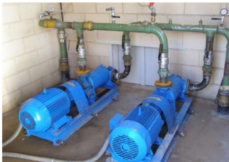
Fig. 6. Hydraulic pumping system consisting of two pumps of 23 kW each.
