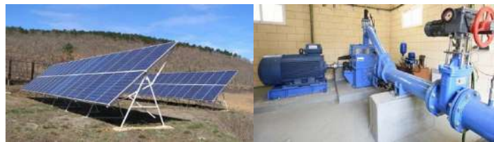
Fig. 1. Photovoltaic turbine zone and Pelton turbine with 40 kW generator.
