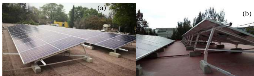
Fig. 8. Solar FV system installed at (a) LAA, (b) ELAU.
