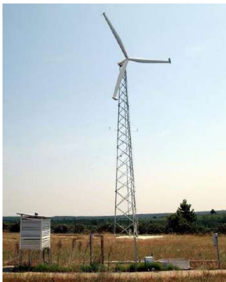
Figure 1. Atlantic AOC Wind Turbine in PEPA I.
